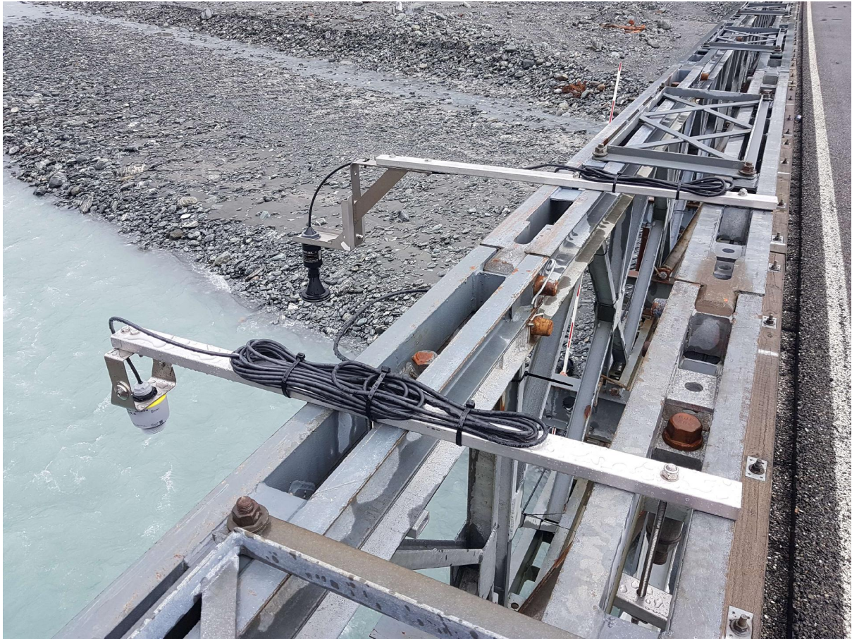
Figure 3: Radar sensors installed over the water of the Waiho River, one new owned by NIWA, one relocated and operated by WCRC.
